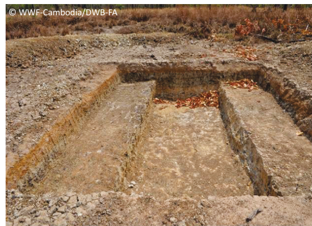
Image 1. Waterhole # 2 following artificial deepening (to depths of 50 and 100-cm; total earth excavated 18-m 3 ) in April 2011.
