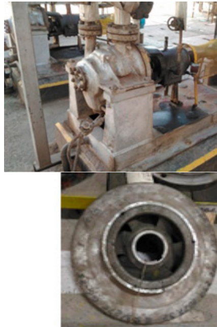
Figure 4. Rotor pump P-502B in a Kermanshah oil refinery.
